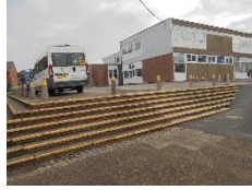
Steps have no handrails
